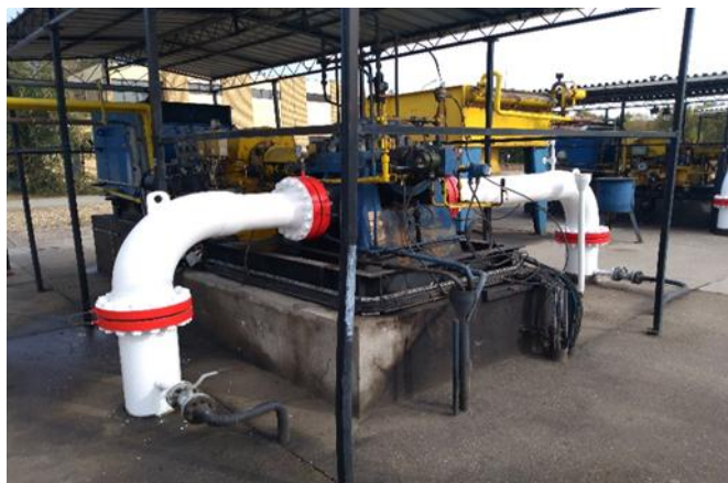
Pumpa za transport sirove nafte.
